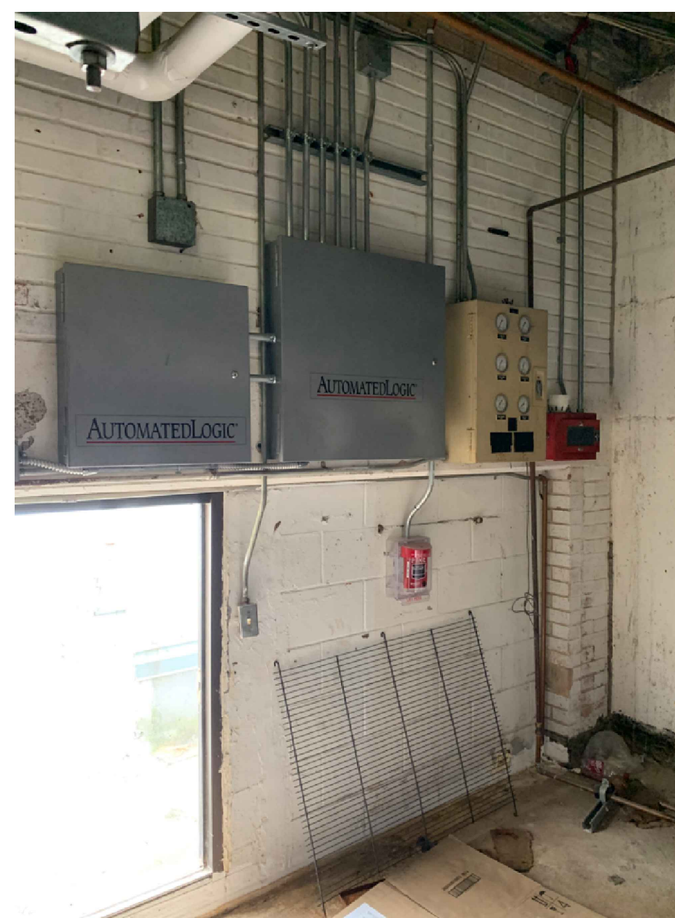
835 EAST LEVEE BUILDING 02 EXISTING HVAC CONTROLS IMAGE SCALE : 1/8" = 1'-0"
