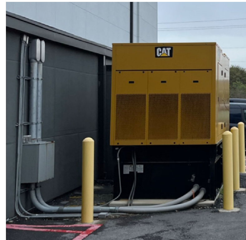
03 EXISTING GENERATOR IMAGE SCALE : NONE
